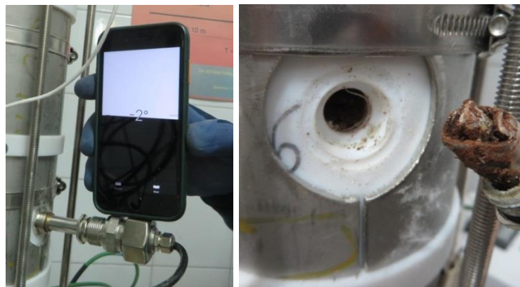
Figure 27 Extraction of sensor RH/T3 and appearance after extraction
